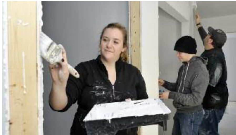
Students Bailey Eberle, Stephen Sharpe, and Andrew Lindenbach gave a Saturday to help with the construction of a Habitat for Humanity home in north central Regina.
